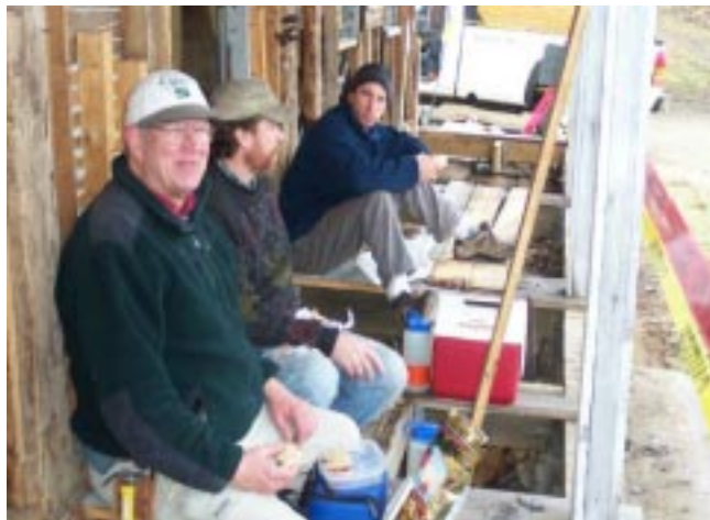
Volunteer Dave Birchenough (left) breaks for lunch with staffers Gary Stansfield (center) and Jesse McNeil (right). SPNHF is in the midst of deconstruction project, in an effort to return the land to its natural state, at SPNHF's Welch Farm forest in Hancock
